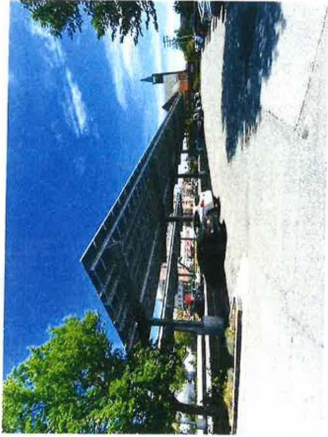
Solar Carport Installation with EV Charging Stations at Village of Patchogue
