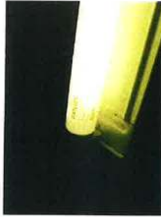
T12 Lighting Village Hall
