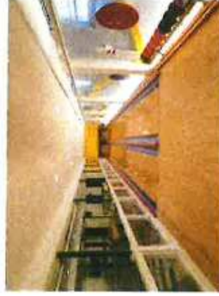
T8 Lighting Community Center
